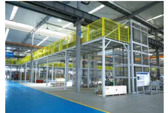
高架物流输送线 Elevated products transport line
